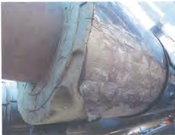
Figure 1. Primary vapour barrier aluminium foil with localised corrosion at the lower half.
